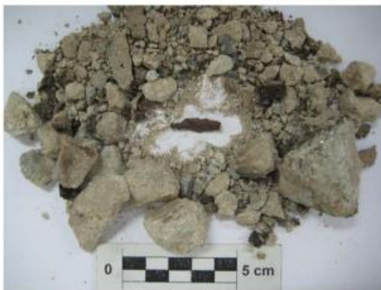
Figure 2: A cyclopean piece of concrete that is held together with a steel nail.
